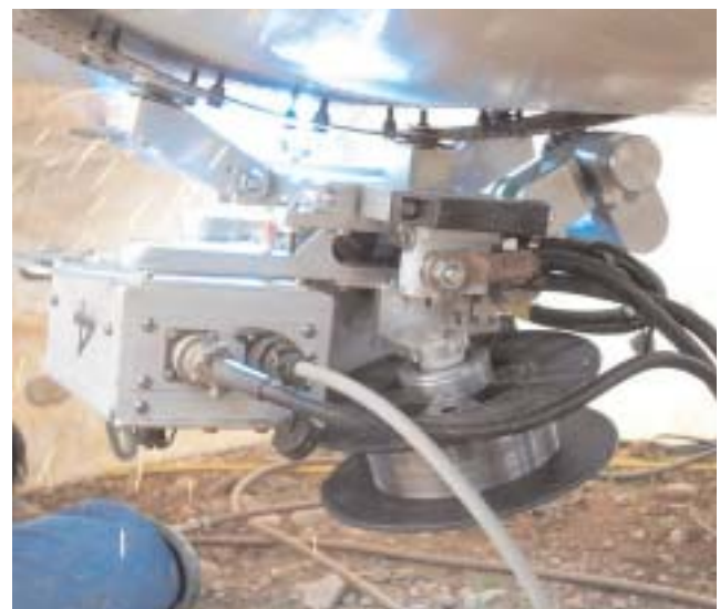
Fig 2. Mechanised uphill welding with rutile flux-cored wire on the X80 Hatton-Silk Willoughby line Photo courtesy of Gridweld Ltd.
